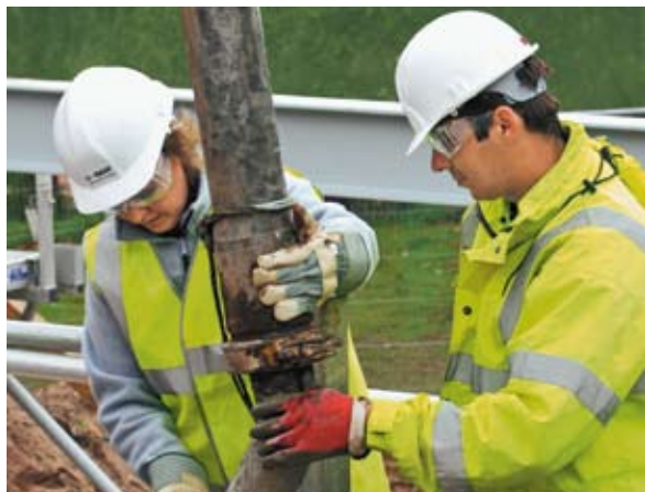
Claire Farrar on site during construction of the low energy house in Nottingham, England, inaugurated in spring 2008.
